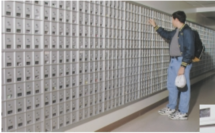
The Student Union building at the University of North Carolina– Greensboro has over 13,000 rear-loading Bommer mailboxes.
